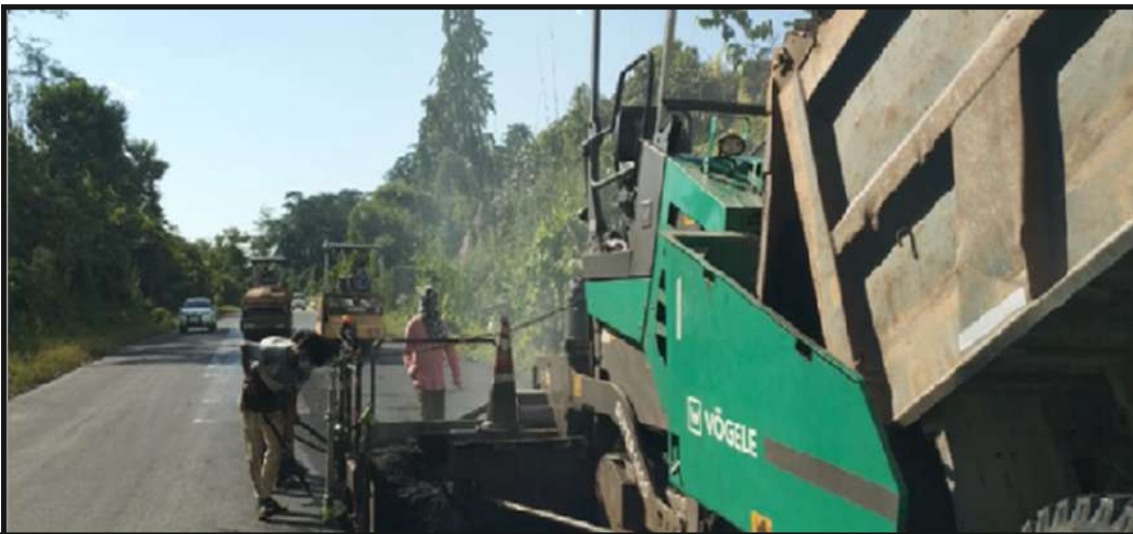
Laying of Bituminous Layer using Plastic Waste on Roing-Koronu-Paya Road in Arunachal Pradesh
