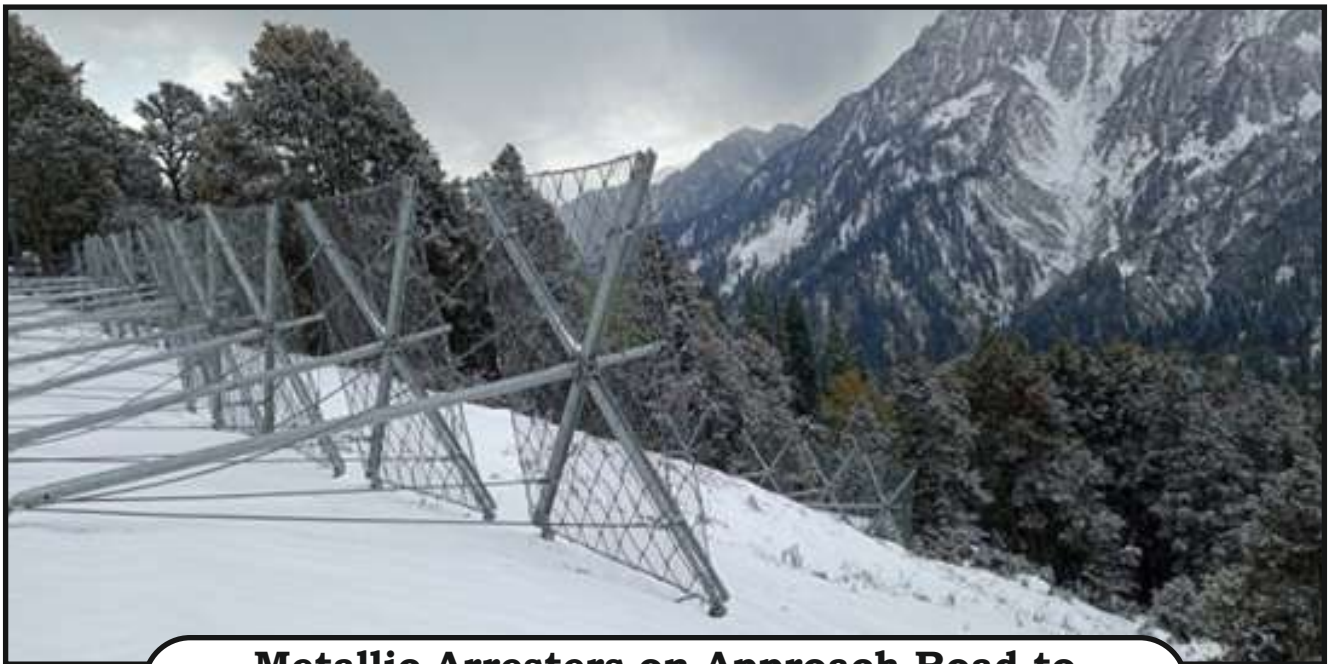
Metallic Arresters on Approach Road to South Portal of Atal Tunnel
